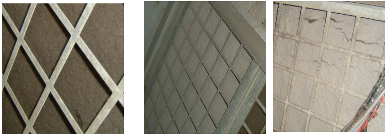
Fig. 14 Evaporator air filter fouling snapshots
