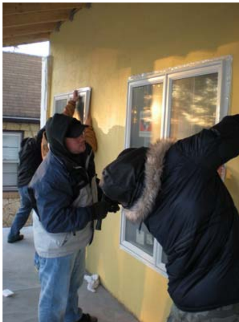
Graduate students add energy efficient windows to the outside of the ZNET house. Courtesy Photo: Engineering Communications
